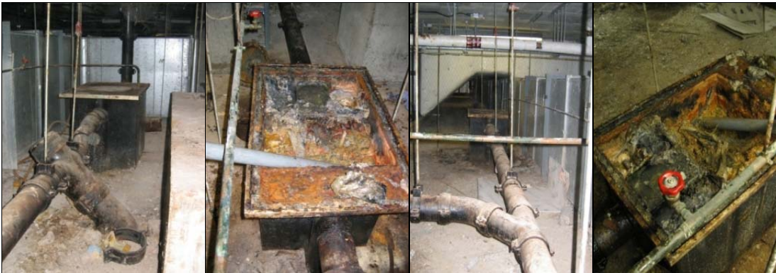
Original mild steel grease traps are vacuum cleaned and waste removed before decommissioning
