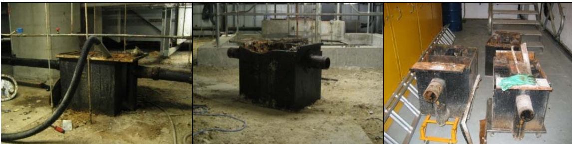
Old units decommissioned and prepared for removal from site and environmental re-cycling
